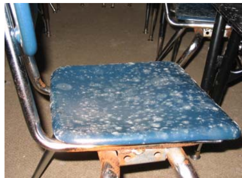
Neil Armstrong Elementary - Hurricane Charley - August 2004 Charlotte County Public Schools, Florida Mirco Assessment Report
